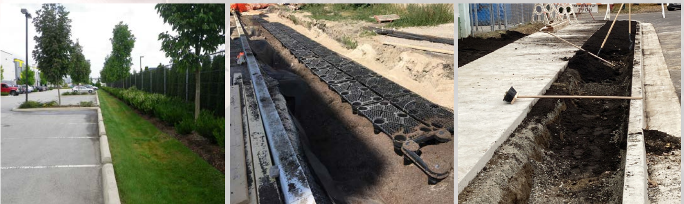
From left to right: Bioswale provides supplemental watering to landscape trees installed in private on-site parking (Surrey) Soil cell installation to extend planting site volume (Winnipeg) Structural soil installation to bridge planting strip with soil behind sidewalk (Vancouver)
